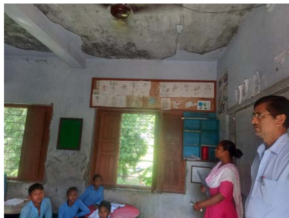
F. Students under damaged ceiling
