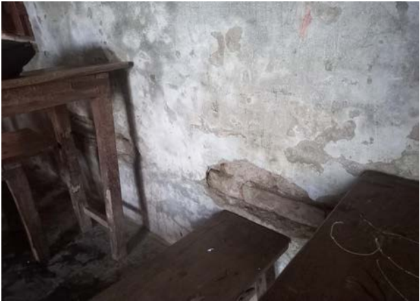
C. Damaged wall
