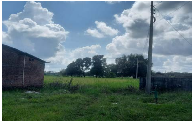
R. Unrepaired school boundary wall due to flood
