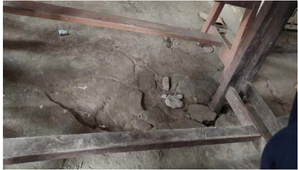
P. Damaged floor at classroom
