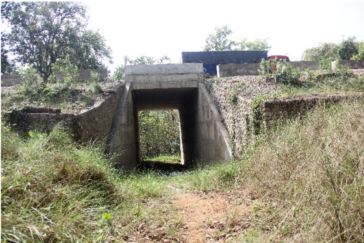
Figure 4: Wildlife underpass constructed at Aaptari of Narayanghat-Muglin highway section in Barandabhar Forest Corridor (Source: Pramod Neupane)
