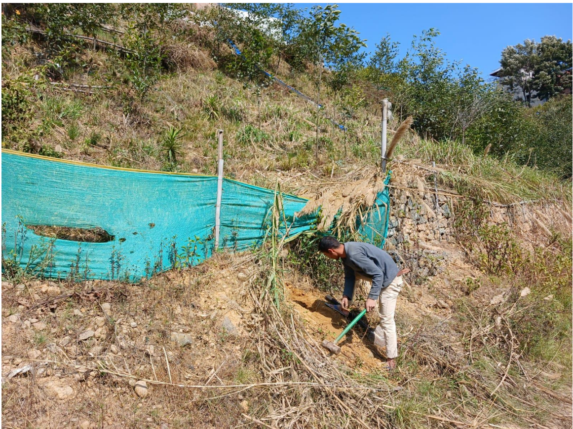
Figure 3-10: Firfire Danda Landslide Image
