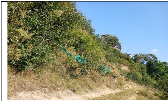
Photo Plate-1: Firfire dada Landslide Site photo
